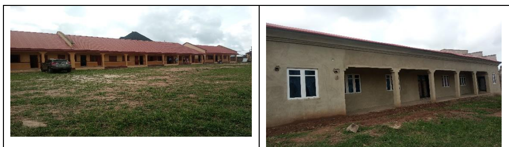
Figure 5 & 6: A block of eleven classrooms and the uncompleted school hall at St Stephen's
